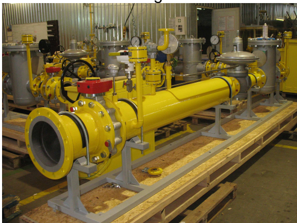
Reduction station at production facility
