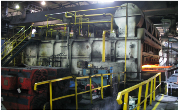
Fig. 11. Furnace before revamping
