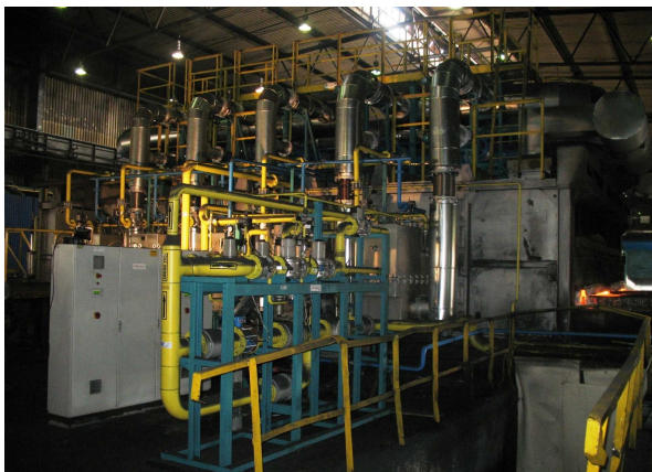
Fig. 12. Furnace and combustion system after revamping
