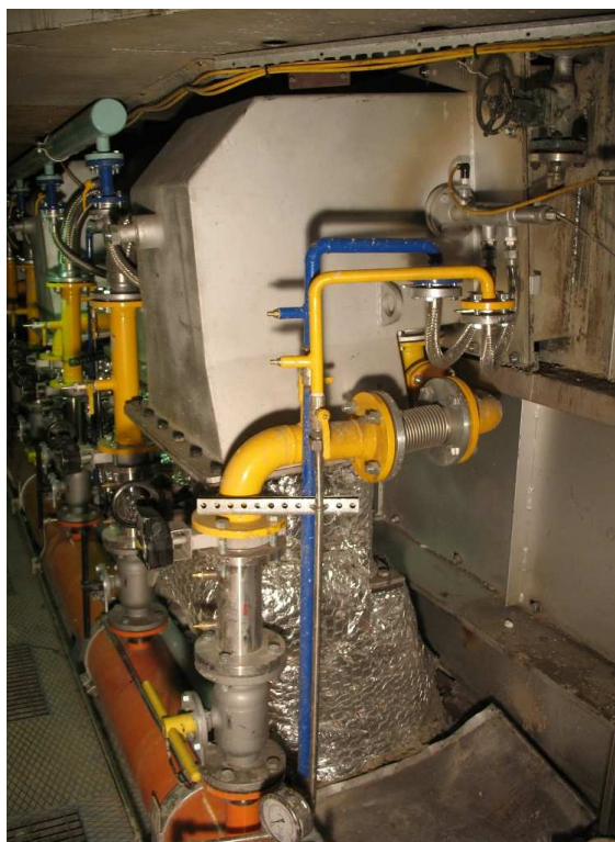
Fig. 1. Photo of the HTB burner with burner piping
