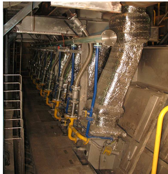
Fig. 6. Photo of the HTB burners, zone 3, SSAB
