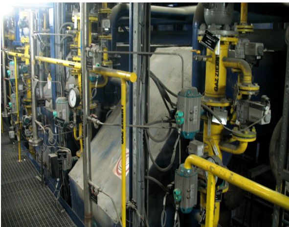
Fig. 6. Part of the final installation – the main burner operating platform
