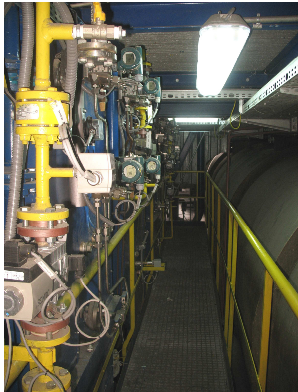
Fig. 8. Part of the final installation – the pilot burner operating platform
