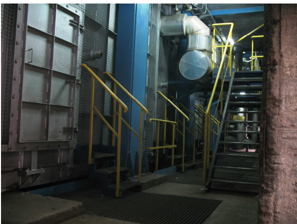
Fig. 7. Part of the final installation – the combustion chamber
