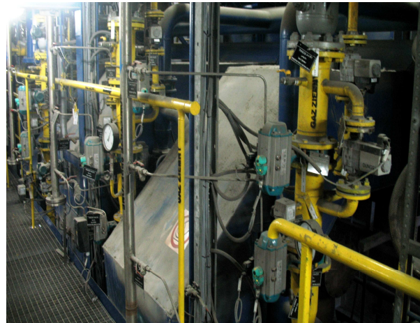
Fig. 20. Part of the final installation – the main burner operating platform
